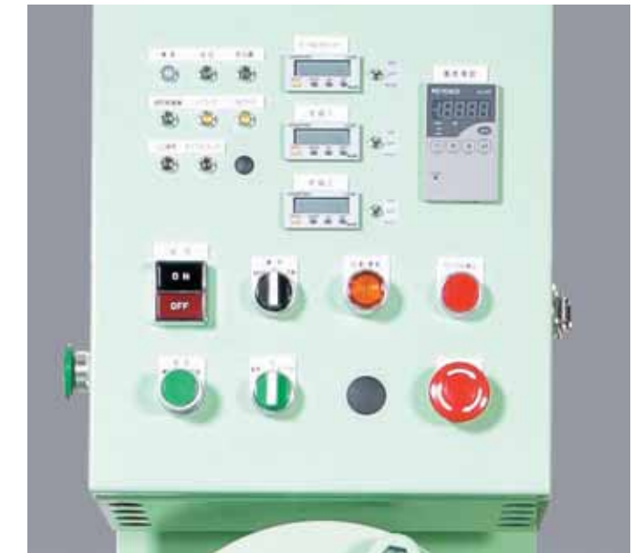
操作盤 / Operation Panel
