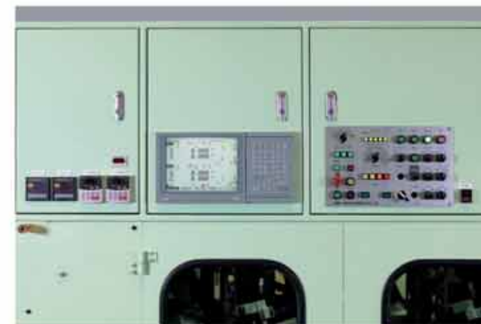
操作盤兼制御盤 / Operation panel (and control panel)
